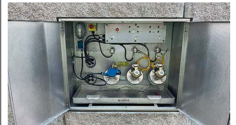
Fernfüllschrank am Bundestag in Berlin Remote filling station at the Bundestag, Berlin designs. In cooperation with Steland Apparatebau, we were able to design and manufacture a remote filling station with special material and design requirements. We were very pleased with the consistently positive feedback from the customer and operator.
